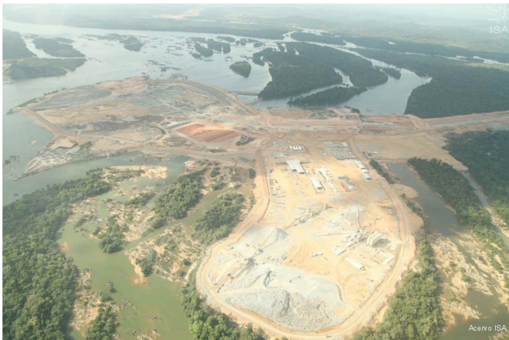
FIGURE 4.12. Aerial view of the Xingu River's local landscape at the Pimental dam building site. Xingu's Big Bend. Note the scope of the river bed, its islands and original vegetation.
